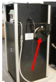
Safety air exhaust (in case of SO 2 leakage)
