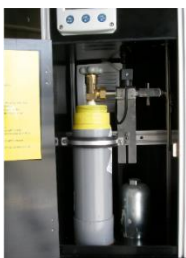
Bottle with SO 2 inside DosiCORR® ED unit
